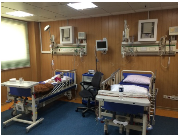
Figure 2. Long-term monitoring room
